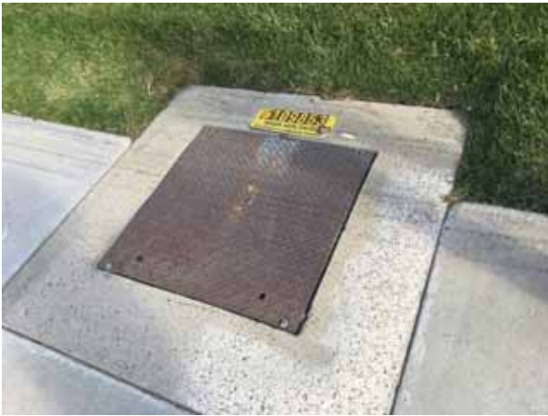
9. View of the subject property: vaulted transformer
