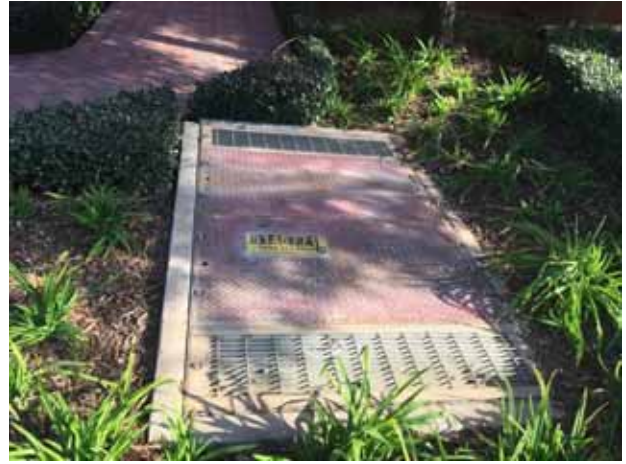
8. View of the subject property: vaulted transformer
